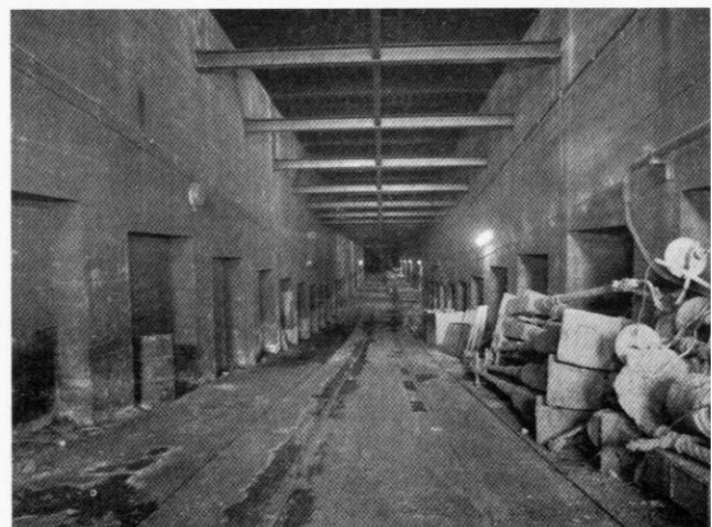
Looking south along the Kingsway tram tunnel towards Holborn station. Photo: Nick Catford
